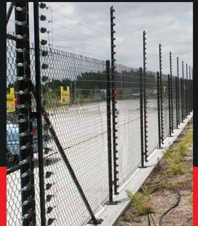
Electric Security Fencing
