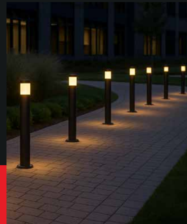
Glowing Pathway Bollards
