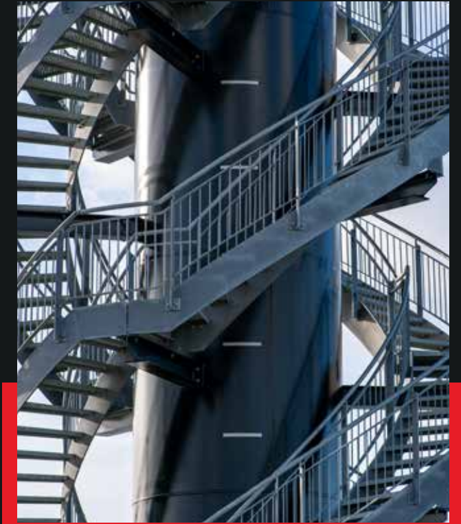
Double Helix Spiral Staircase
