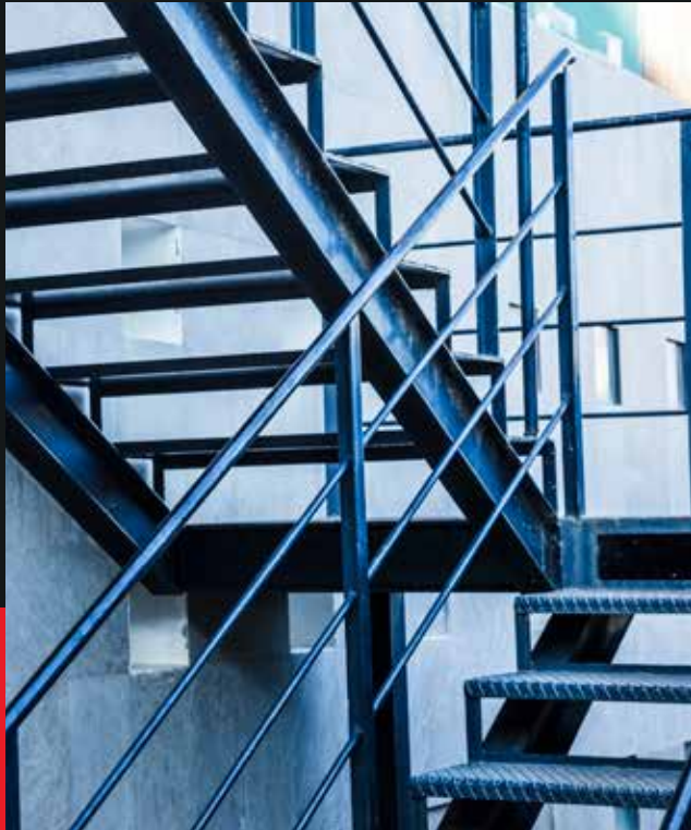
Emergency Exit Staircase
