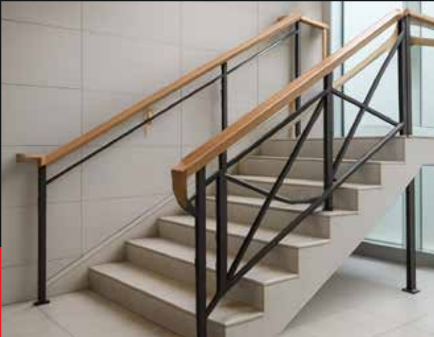
Custom Stair Guardrail
