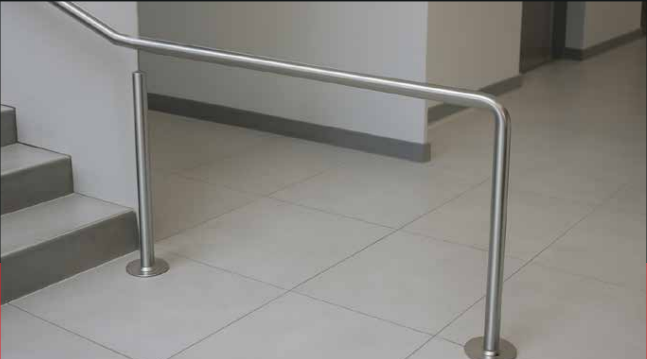
Single Rail Handrail
