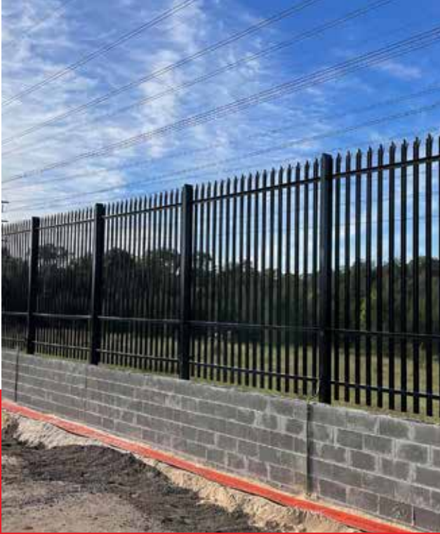
Steel Security Fencing
