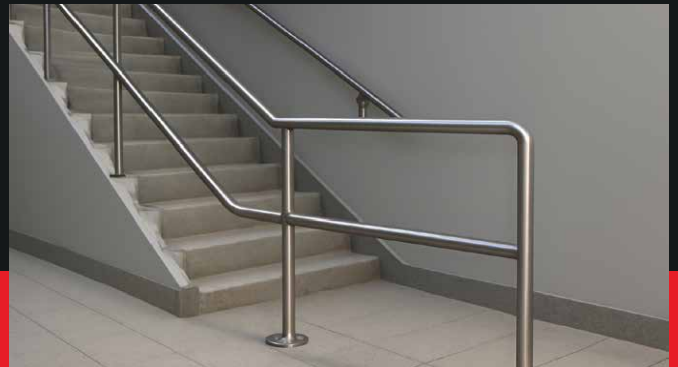
Double Rail Handrail
