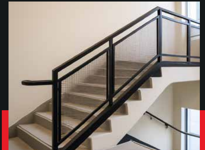
Mesh Stair Guardrail
