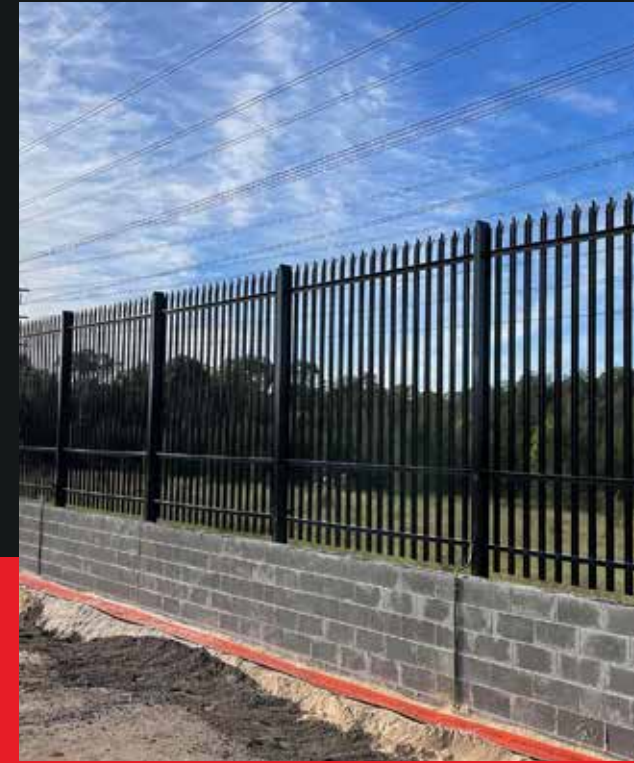
Steel Security Fencing
