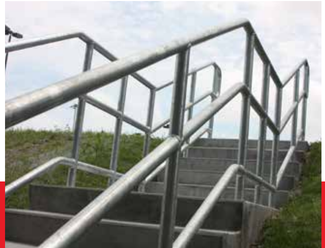
Galvanized Steel Railings
