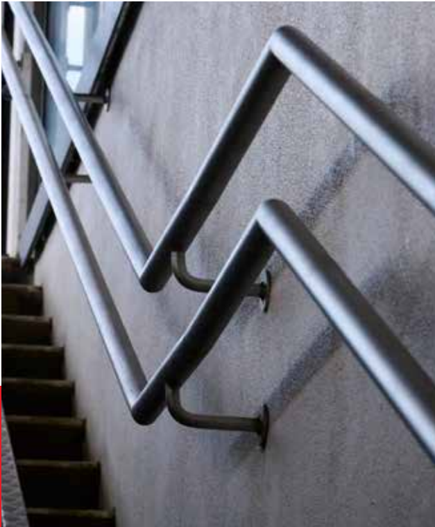
Continuous Pipe Handrails
