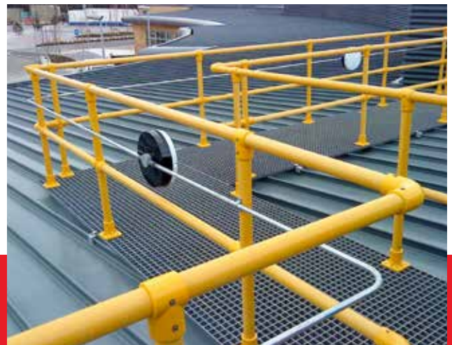
Industrial Safety Rails
