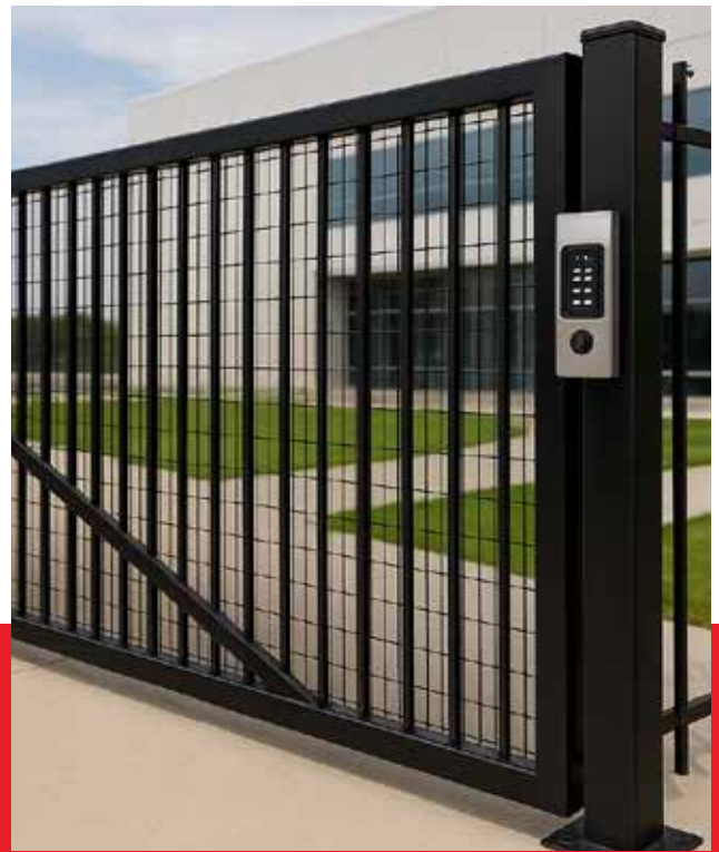
Access-Controlled Security Gate
